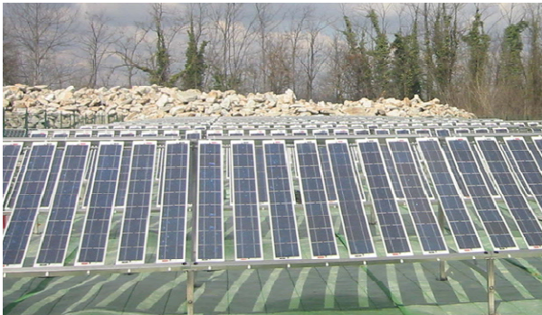
Fig. 8. In foreground liquid cooled PV panels.
